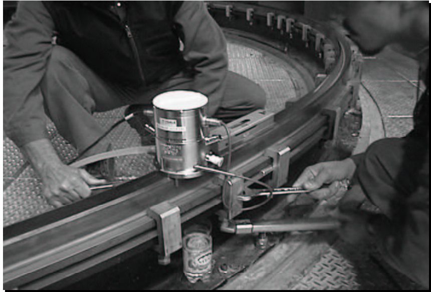
Fig. 6: Azimuth axial track alignment operation (Fogale level system)
