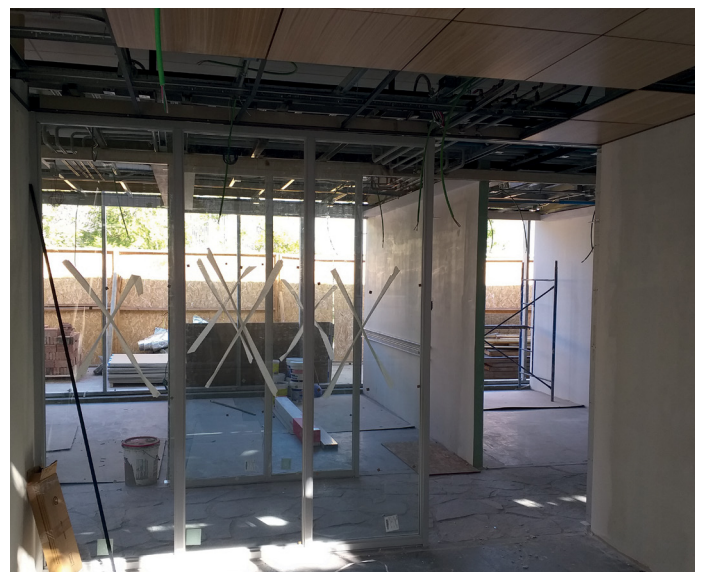
The extension of the main office building at the ESO premises in Vitacura, Santiago will provide 12 new offices.
