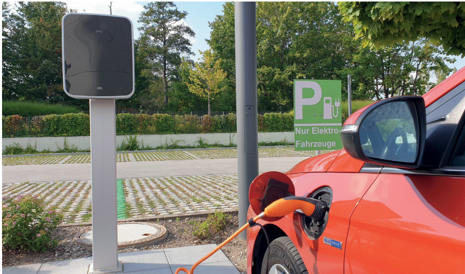
Electric car charging station at ESO Headquarters.
