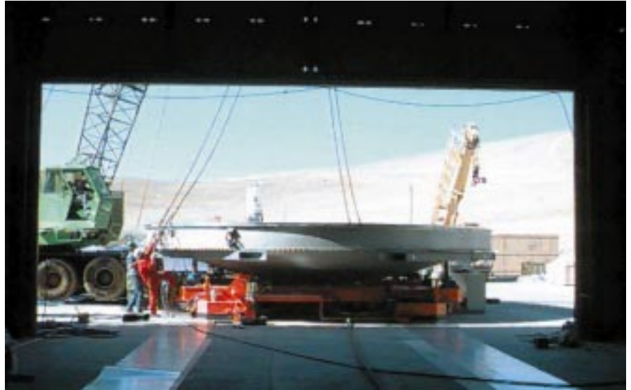
Figure 3: View from the inside of the Mirror Maintenance Building through the 10-m door. The lower part of the coating plant has been placed on the air cushion transport system which will move it along the two tracks seen in the foreground. The total moving weight with an 8.2-m mirror in the chamber is about 50 tons.
