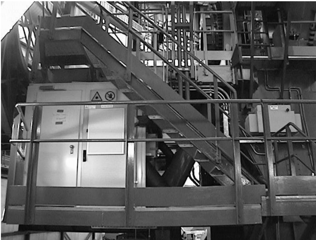
Figure 3: LCR side view, mounted on board of VLT-UT4 under the Nasmyth A platform. The coded access door and the air handling unit control cabinet are seen in this picture.
