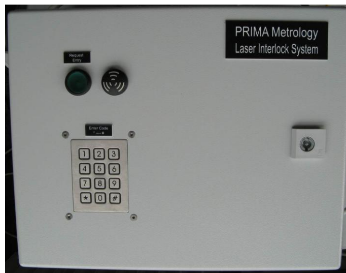
Figure 7 Distributed I/O Cabinet
