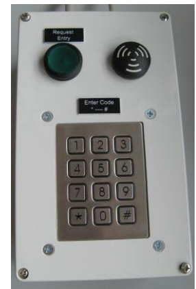
Figure 8 Entry Request / Code Access box
