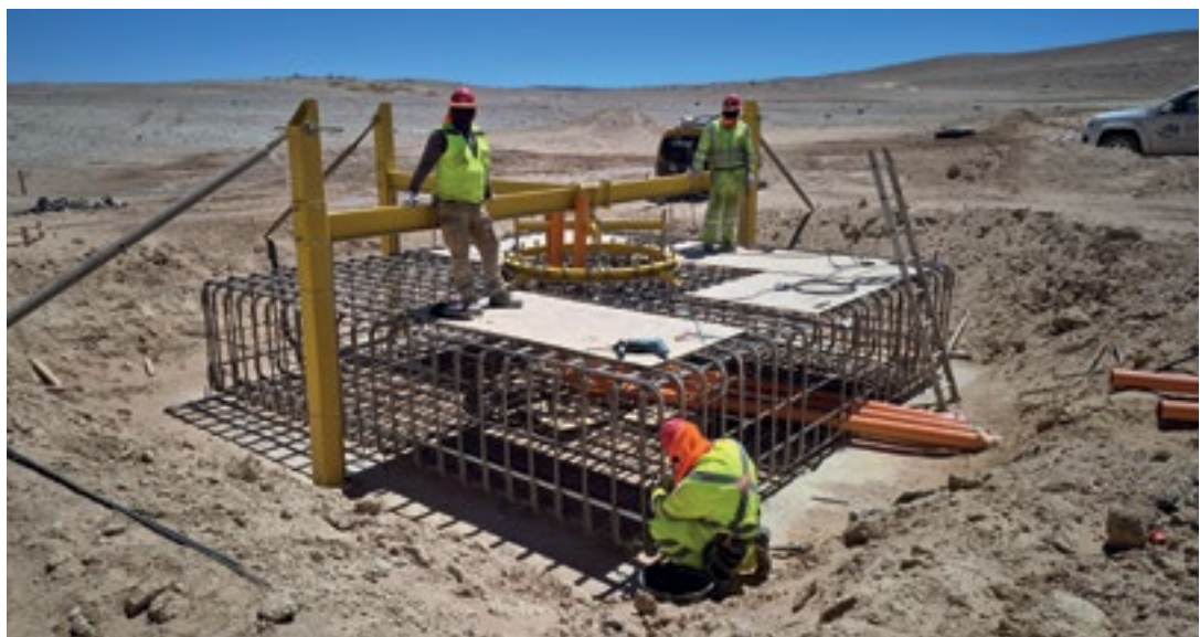
Construction of one of the telescope foundations for the 'alpha configuration' of CTAO-South.
