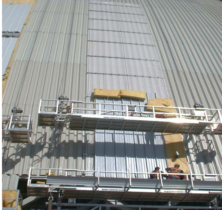
Figure 15-8 lifting platform for inspection and maintenance of cladding
