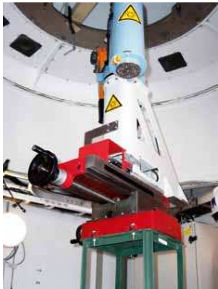
Figure 3. ACD#1 during installation in the antenna receiver cabin.
