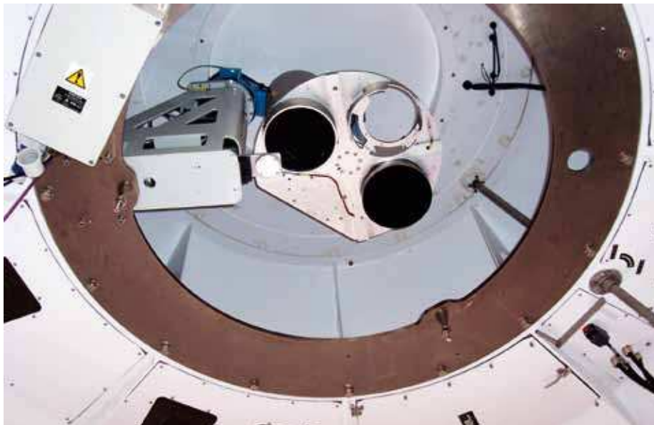
Figure 4. ACD#1 installed in a MELCO antenna.
