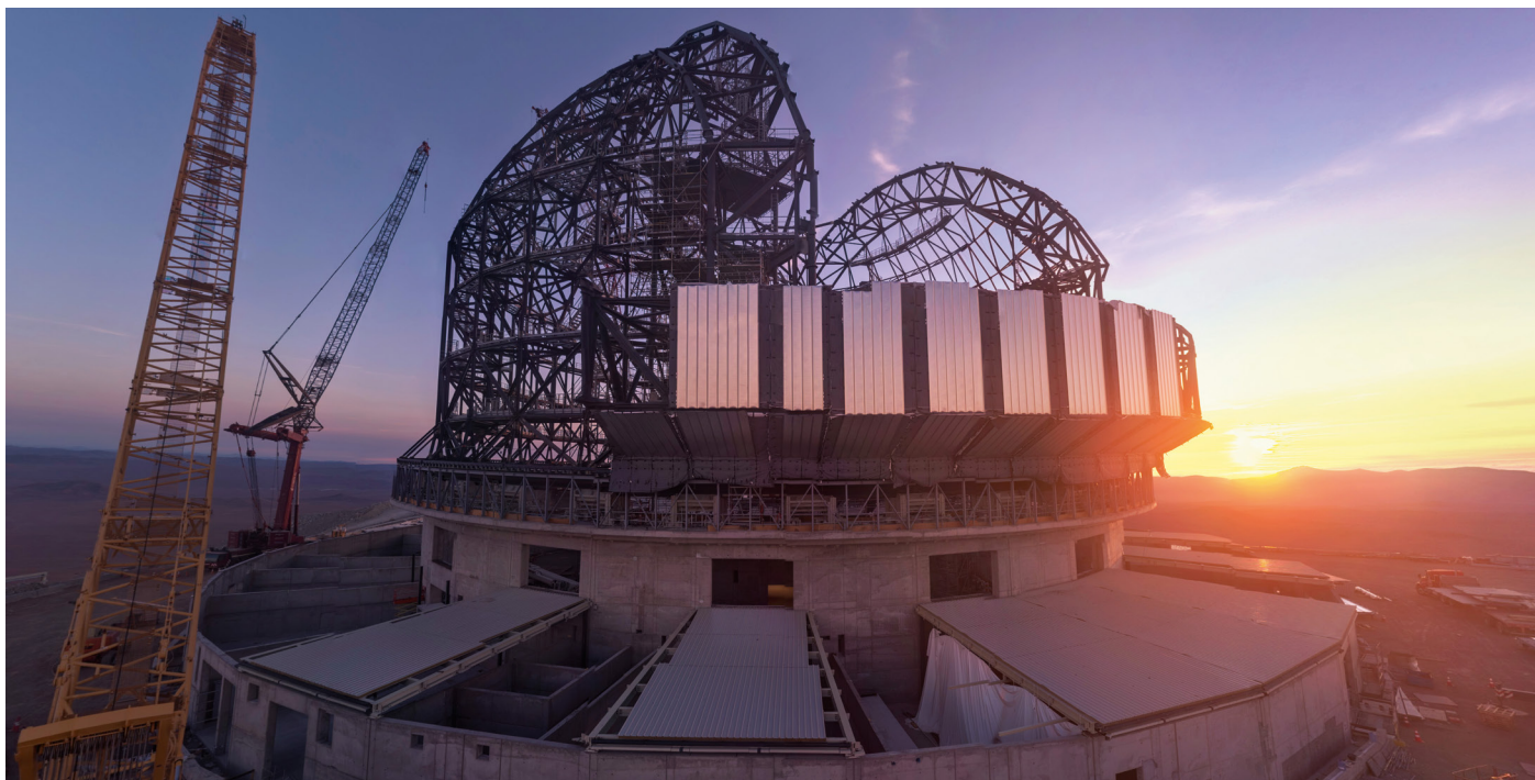
ESO's Extremely Large Telescope (ELT) is quickly coming together before our eyes. In this webcam image over Cerro Armazones in Chile from 16 February 2024, the setting Sun illuminates the first pieces of cladding installed on the ELT dome. The hemispheric structure
