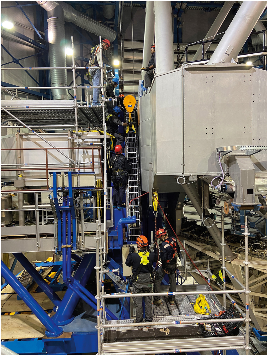
Figure 7. Implementing the upgraded cable wrap at Nasmyth B on UT2 in June 2023.
