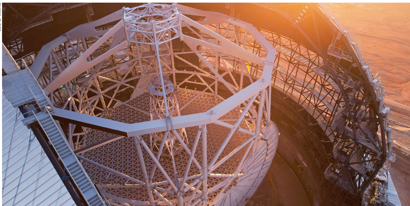
Bathed in the sunset light of Chile's Atacama Desert, this image shows steady progress in the construction of ESO's Extremely Large Telescope (ELT).
