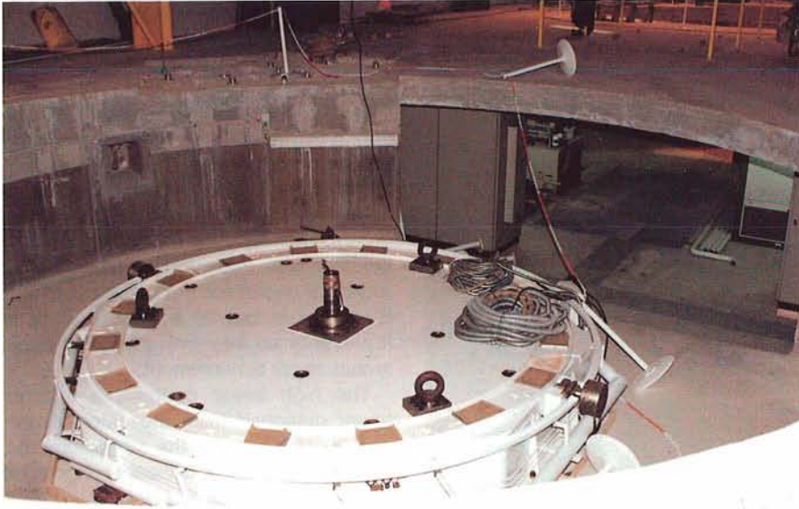
Figure 4: Base of the polishing rotating table installed in its pit. The oil pads at the periphery of the table base are protected by grey yellowish plastic. The track is attached to the table.
