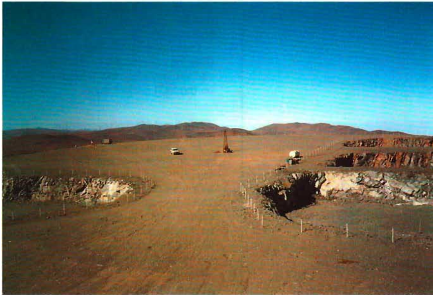
Figure 5: Overview of the Observatory site showing the telescope excavations and, in the centre of the "Platform" the equipment used to measure the GVTF. The view is taken from the north.
